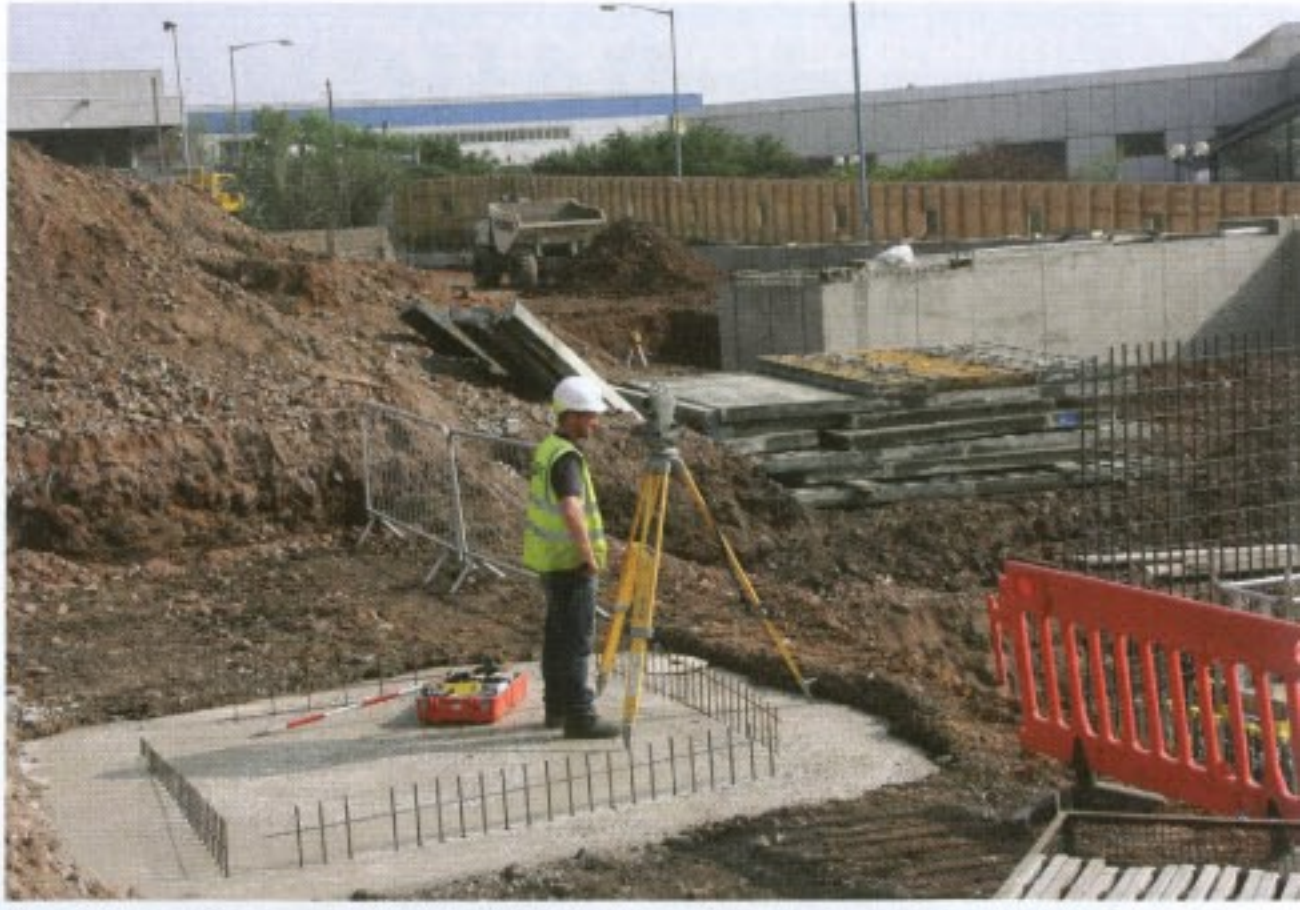
This Picture and Above: PGC's work on site includes constructing the underground car park and base plate work for the vertical stanchions for the new cash & carry building.
